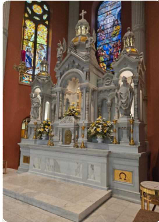
High Altar restoration and cleaning, before and after. The project required special narrow-gauge scaffolding to reach all areas.
