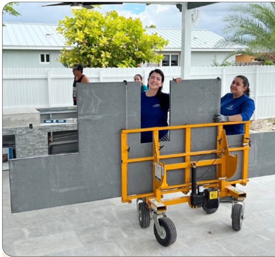
The No Lift expands the labor pool, enabling women to join the ranks of highly skilled slab installers, something utterly unheard of in the past.
