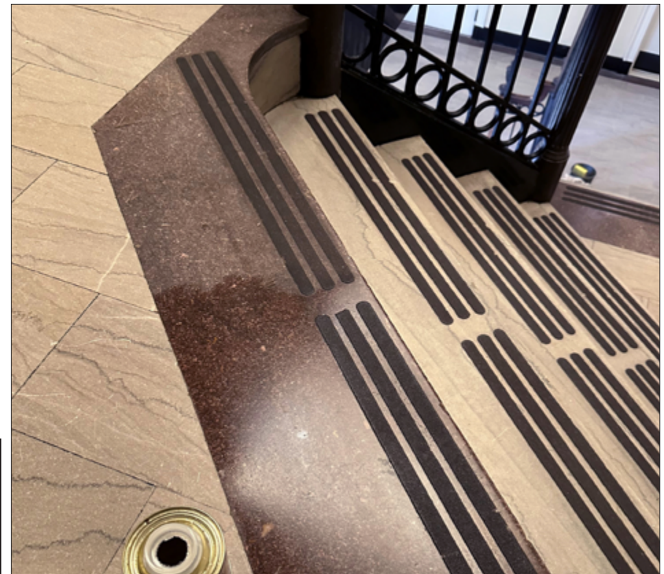
Tennessee Pink Marble stairs after coating removal. Tenax Ager was applied to the Dark Pink Tennessee marble to restore the deep, rich contrast.
