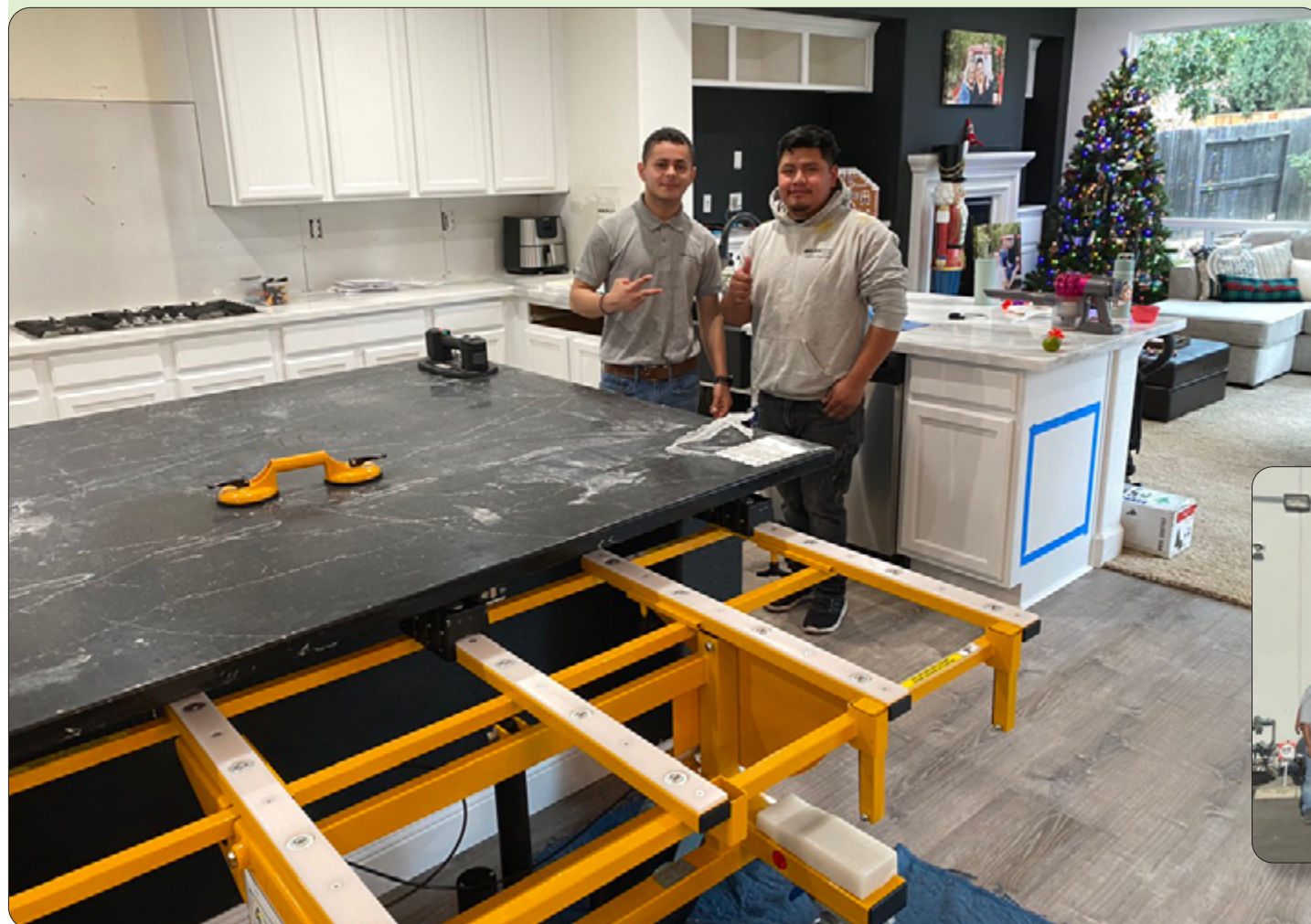
A Block Tops installer team from the Anaheim office moves a full size island into place with their No-Lift Cart.
