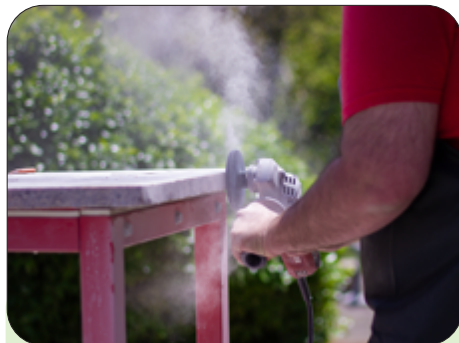
Proper masking and wet fabrication are part of managing dust from cutting, grinding and drilling stone.
