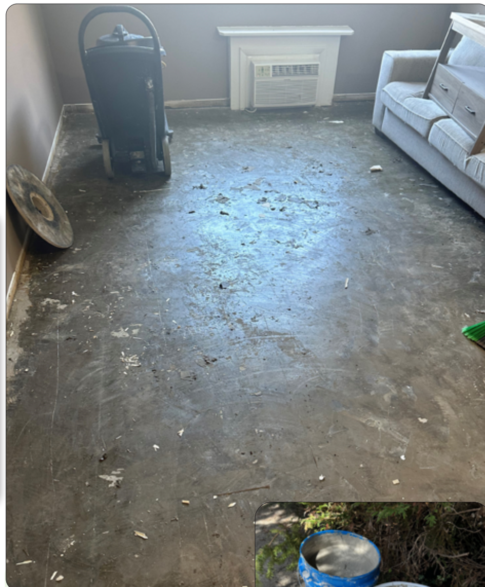
Underneath a layer of vinyl plank flooring, the concrete floor was overlaid with multiple layers of different adhesives.
