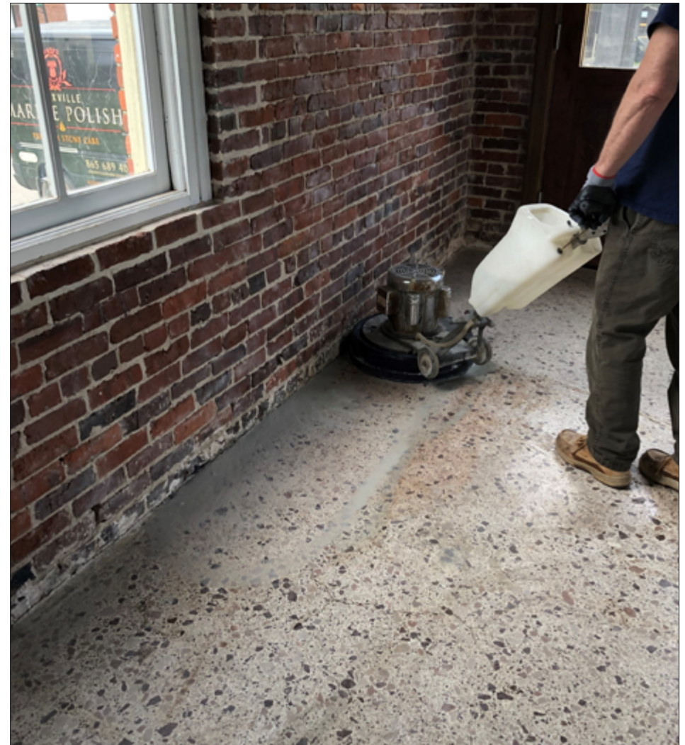
Refinishing a cement-based terrazzo floor. Older terrazzo installations are more likely to have a cementitious binder instead of an epoxy binder and will affect your tool choices.
