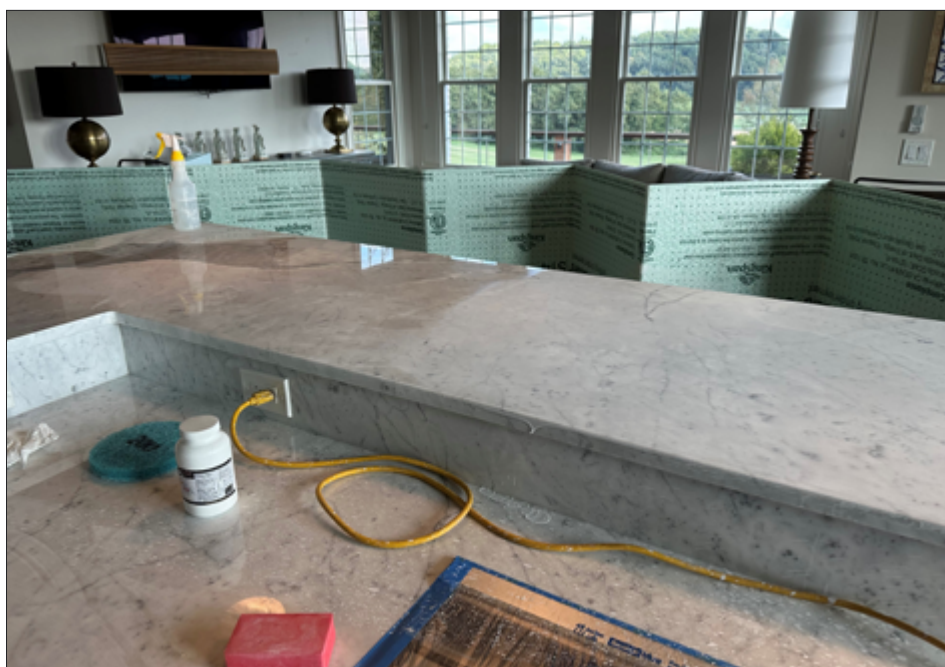
Test area completed on center island, where the 100 grit honed finish was decided. Notice the partition wall (foam core board) and the masking on the range.
