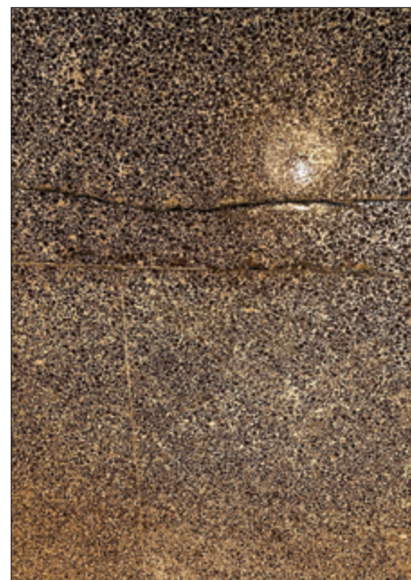
Damage also included shifting eruption in the door threshold.
