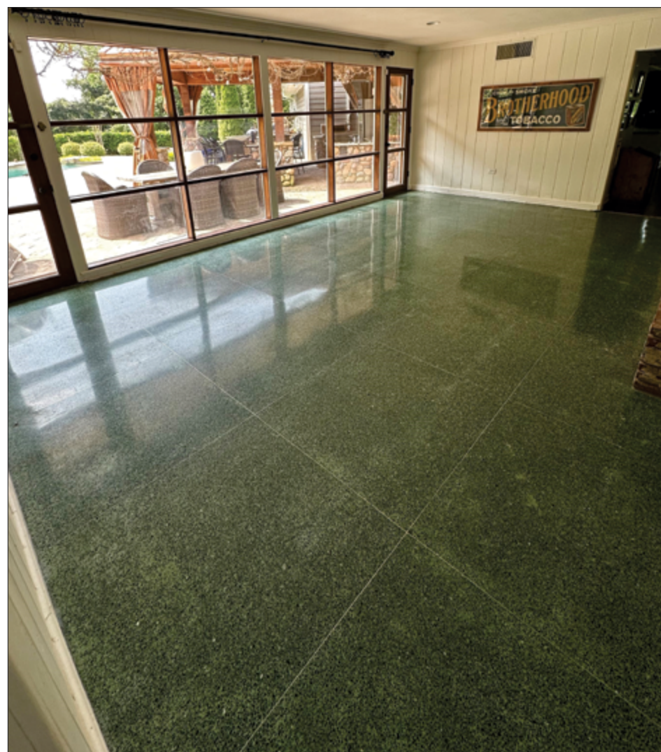
So, with grind marks, blade cuts, cracks and settling issues, the coarse grind with the 40 grit was totally necessary. Considering the issues on these floors, the project turned out really nice and the client was very satisfied with the results.
