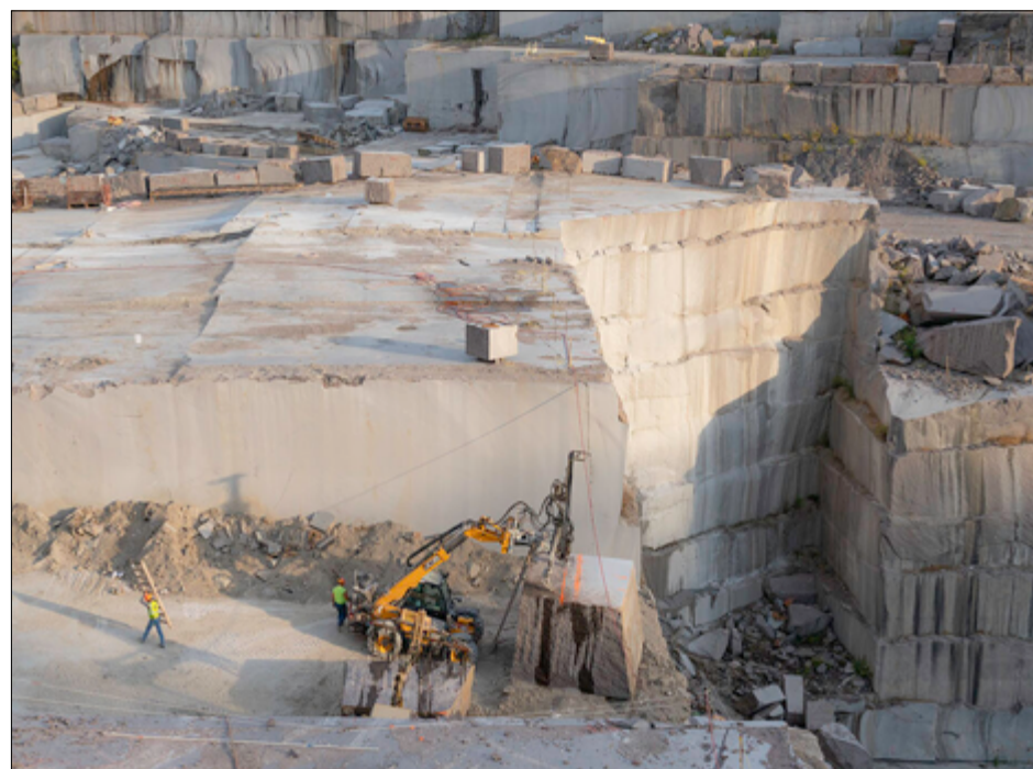
Early morning work at the quarry: extracting a block from the working face
