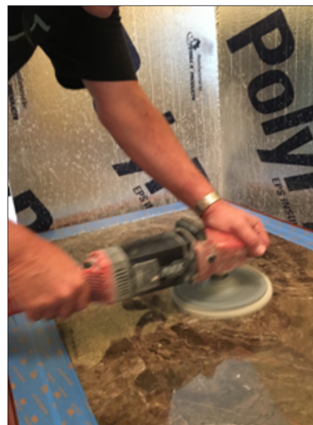
Refinishing a table top on site, and using foam board insulation walls and blue tape to protect the surrounding area.
